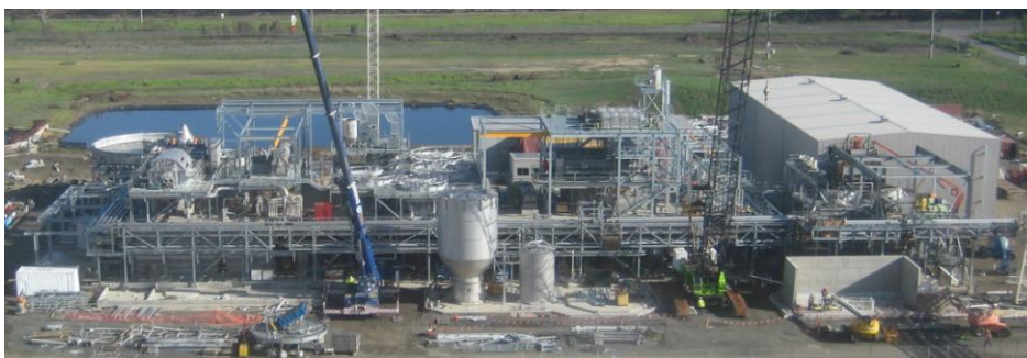
Figure 12. In 2013 Australian Paper began construction of a $90 million paper recycling plant at Maryvale in Victoria, to increase substantially the production of local recycled paper
